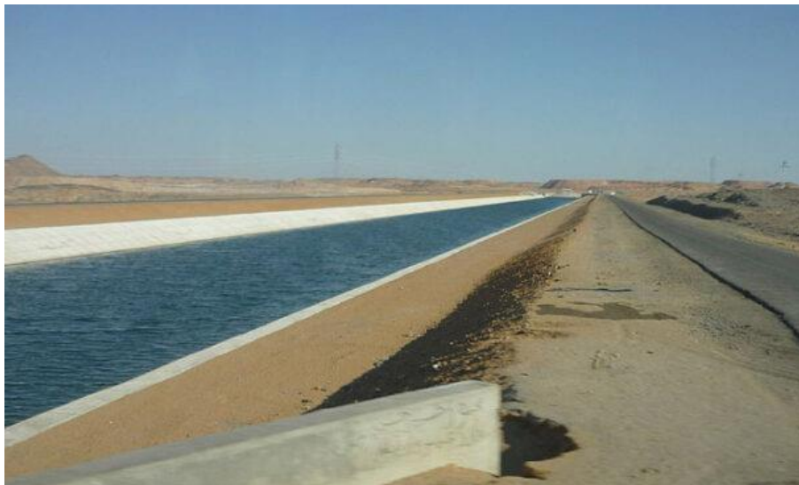
View of the canal delivering water from the Nile to the Toshka Lakes (photograph: Rémi)
